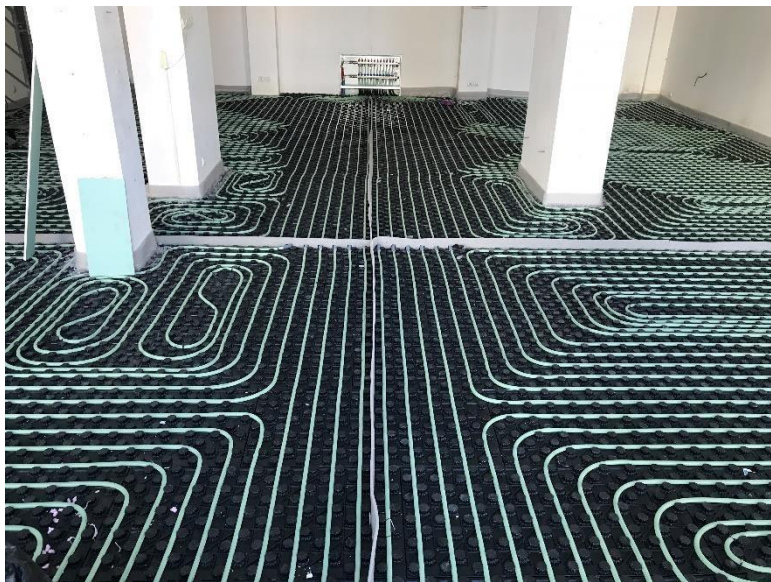
Instalatii incalzire in pardoseala
